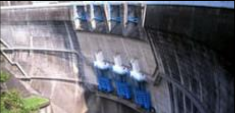
IHI Infrastructure Systems watergates
