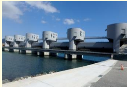
Flow control watergates (MLIT and local governments)
