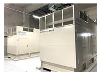
Gas turbines (GT)
