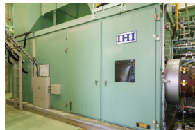
2,000 kW-class ammonia co-firing gas turbine
