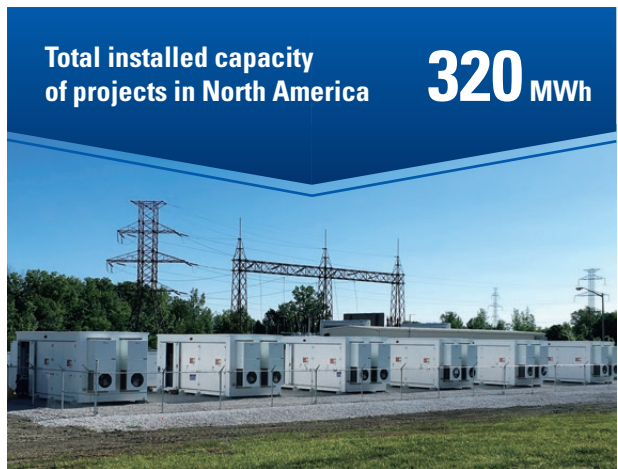
Project in Sarnia, Ontario (Battery Energy Storage System)
