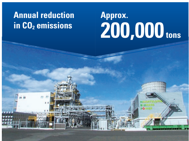
Nanatsujima Biomass Power Plant
