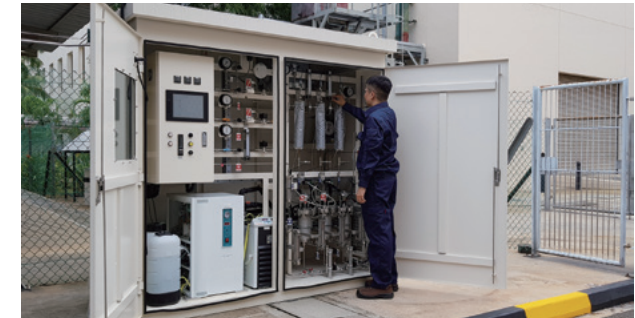
Demonstration Plant for Methanation Technology Installed in ISCE 2
