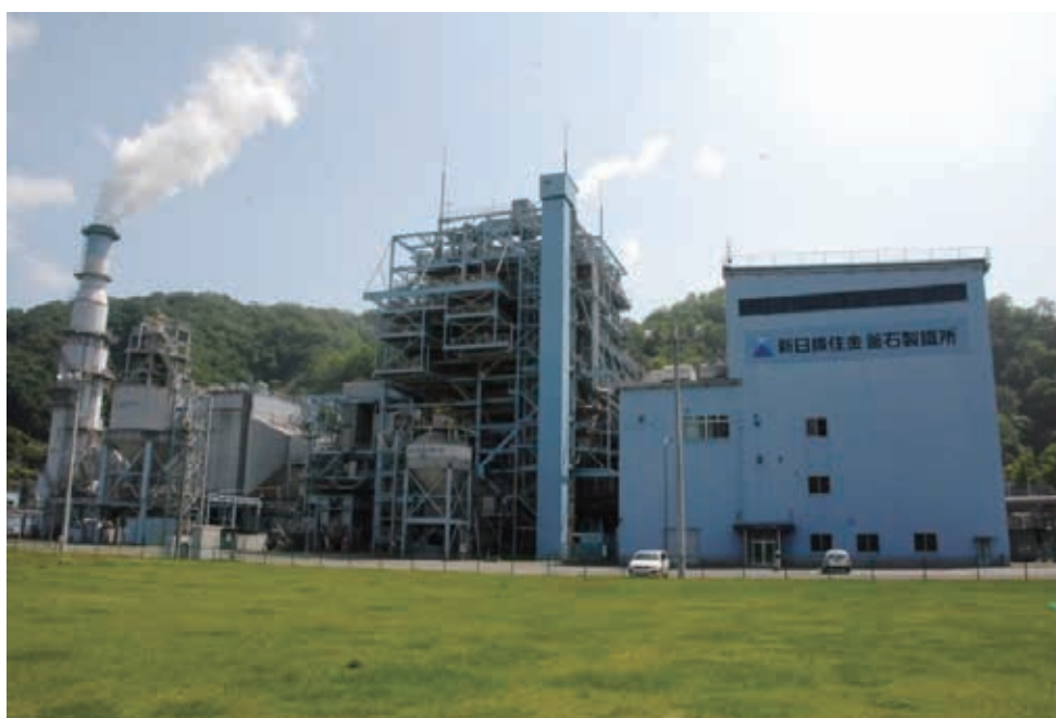
149 MW coal-fired thermal power plant at Kamaishi Works of Nippon Steel & Sumitomo Metal
