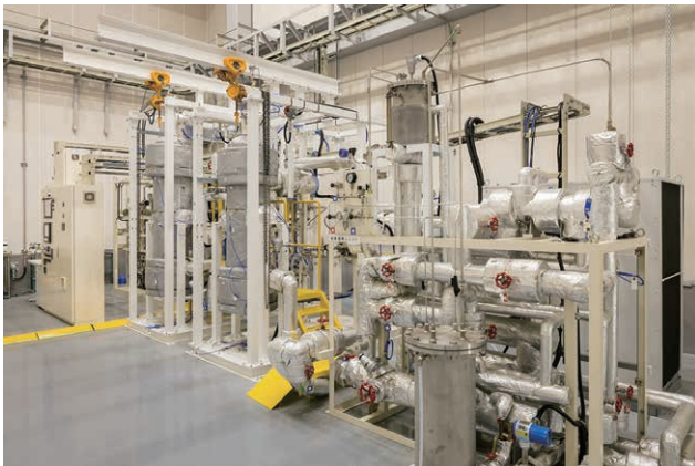
Methane synthesis test equipment installed in Cell No. 1
