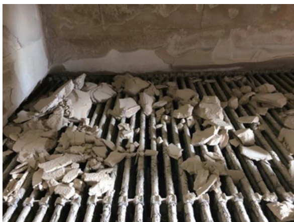
Ash deposits that dropped on the heat transfer surfaces
