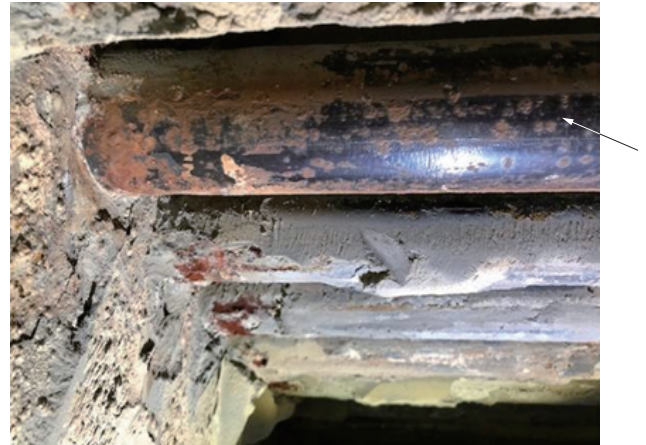
Heat transfer tubes around the GAH inlet (The arrow indicates the tube from which ash deposits have been removed.)
