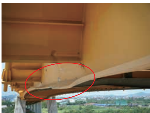
Fig. 5 Steel girder damage (outer side)
