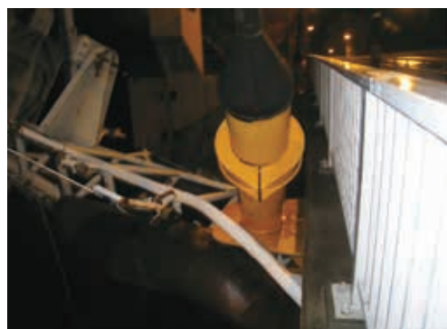
Fig. 3 Close-up photograph of damaged part
