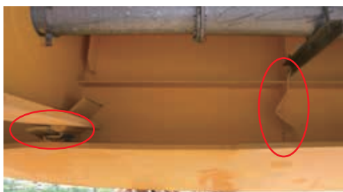
Fig. 9 Buckling of stiffeners
