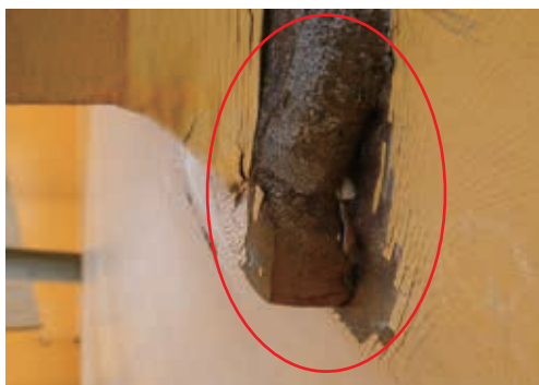
Fig. 8 Crack in web plate
