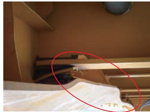
Fig. 6 Steel girder damage (inner side)
