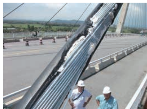
Fig. 7 Stay cable damage
