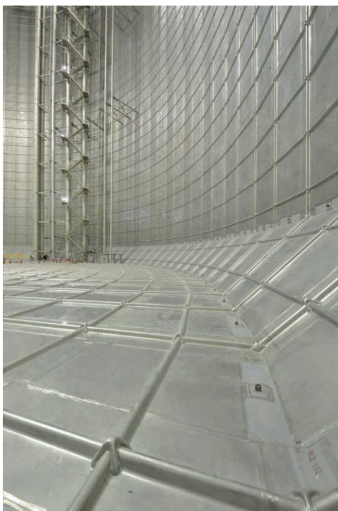
250 000-kL underground LNG tank at Ogishima Plant, Tokyo Gas Co., Ltd. (Photo provided by Tokyo Gas Co., Ltd.)
