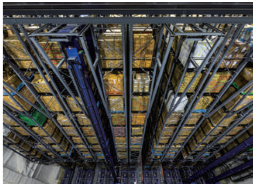
Freezer automated storage and retrieval systems
