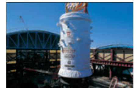
Reactor pressure vessel Photo courtesy of Tokyo Electric Power Company Holdings, Inc.
