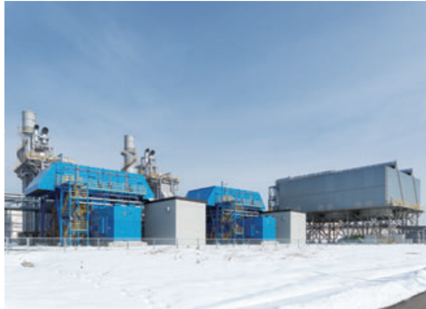
LM6000 gas turbine power plant
