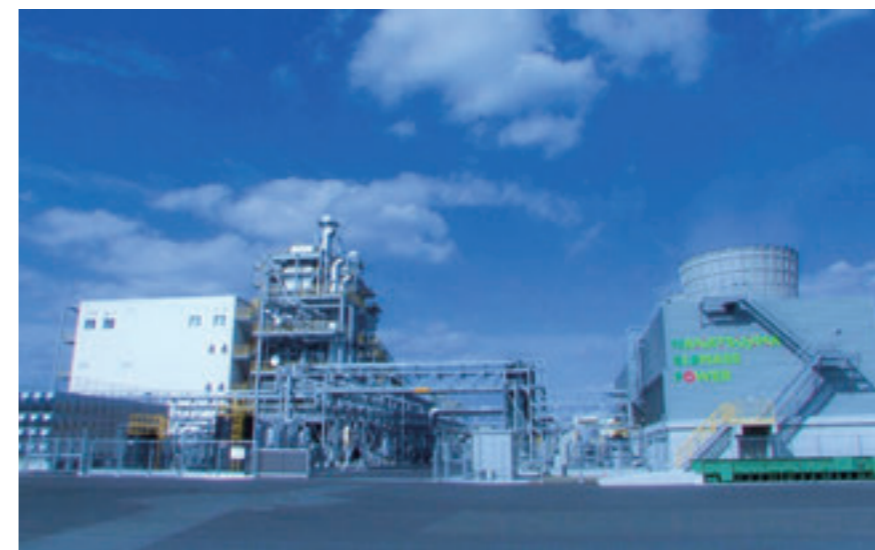
Biomass combustion technology Photo courtesy of Nanatsujima Biomass Power Limited Liability Company
