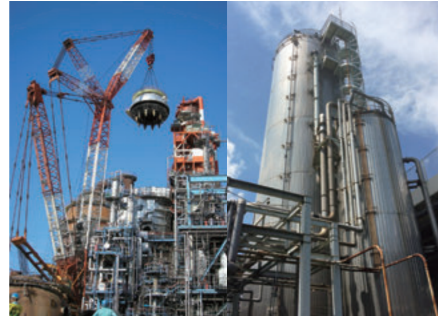
Pressure vessels / Wastewater treatment facility
