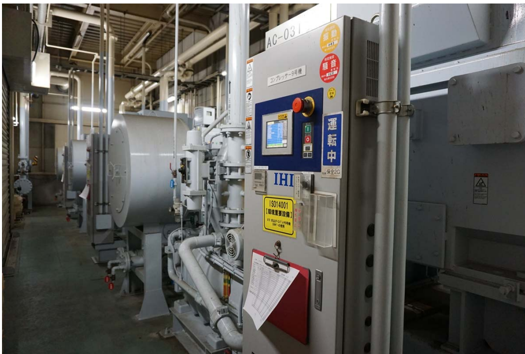
3 units of "TRA series" centrifugal compressors (400kW)
