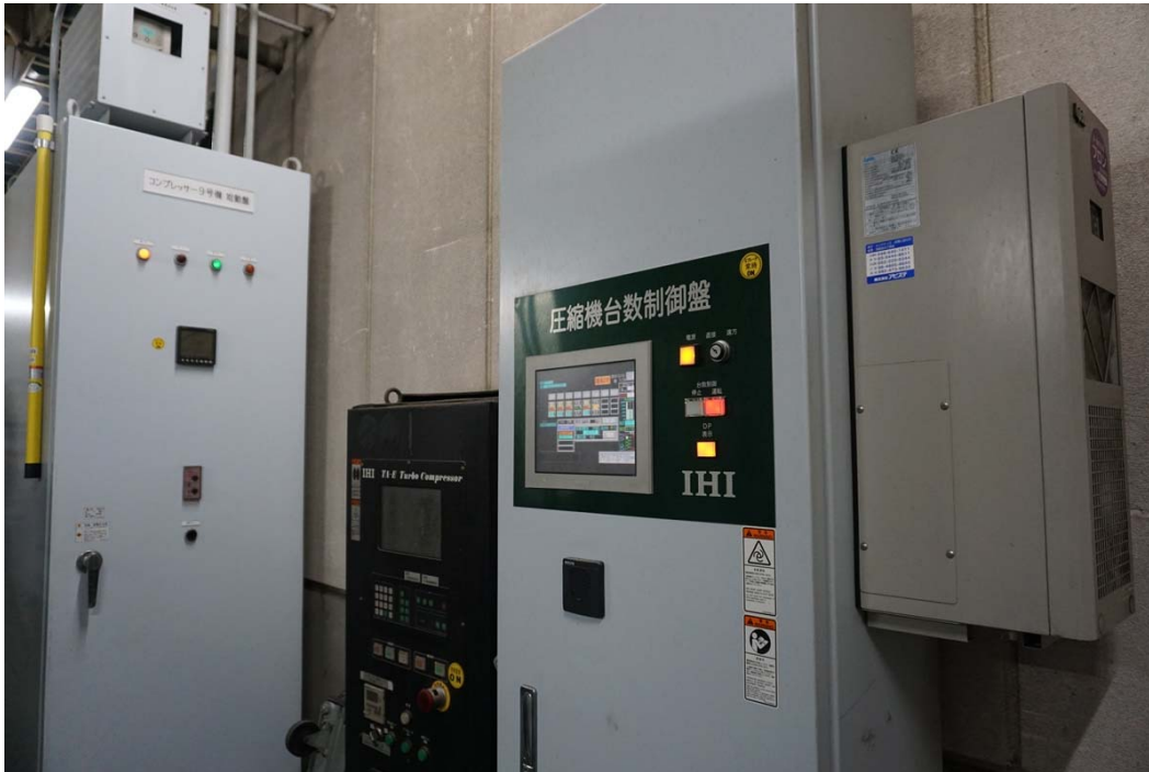
IHI Group control panel
