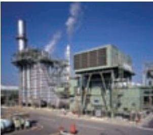
LM6000 gas turbine combined cycle power plant
