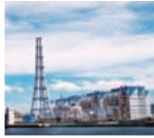
Boilers for power plants
