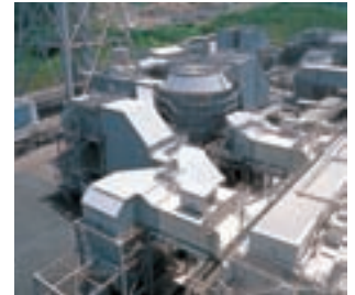
Air pollution prevention systems
