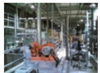
Wastewater treatment system at Soma No. 2 Aero-Engine Works
