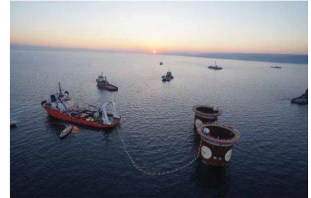
Positioning the main tower foundation caissons and sinking them onto the seabed
