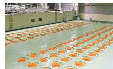
Source : Japan Nuclear Fuel Limited Vitrified waste storage facility
