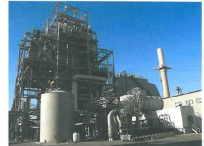
Biomass power plant, United States (Rio Bravo Fresno)
