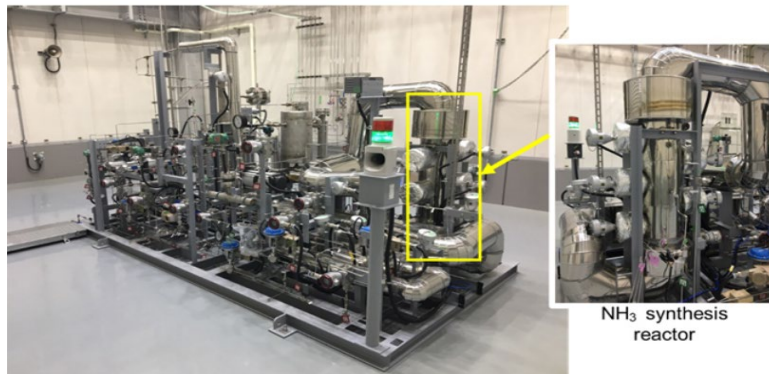
<Green ammonia production test unit (left) and reactor>
