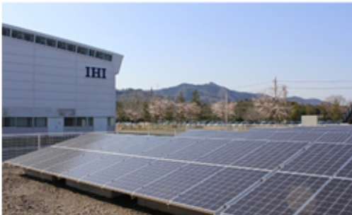
1.1-megawatt solar power system installed in FY2012
