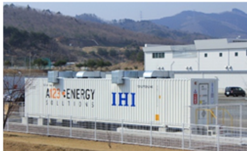
Large 2.8-megawatt-hour lithium-ion battery storage system installed in FY2013
