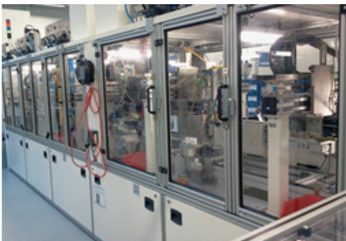
IHI Charging Systems International Germany GmbH's automated production line for vehicular turbochargers equipped with picking robots
