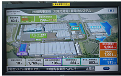
Monitor showing solar power-generation and lithium-ion battery-storage levels.
