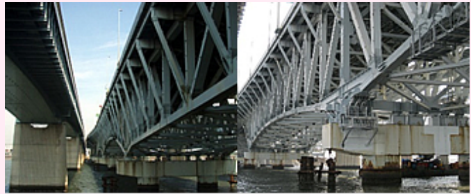
Arakawa Wangan Bridge (on right) before work Arakawa Wangan Bridge after work
