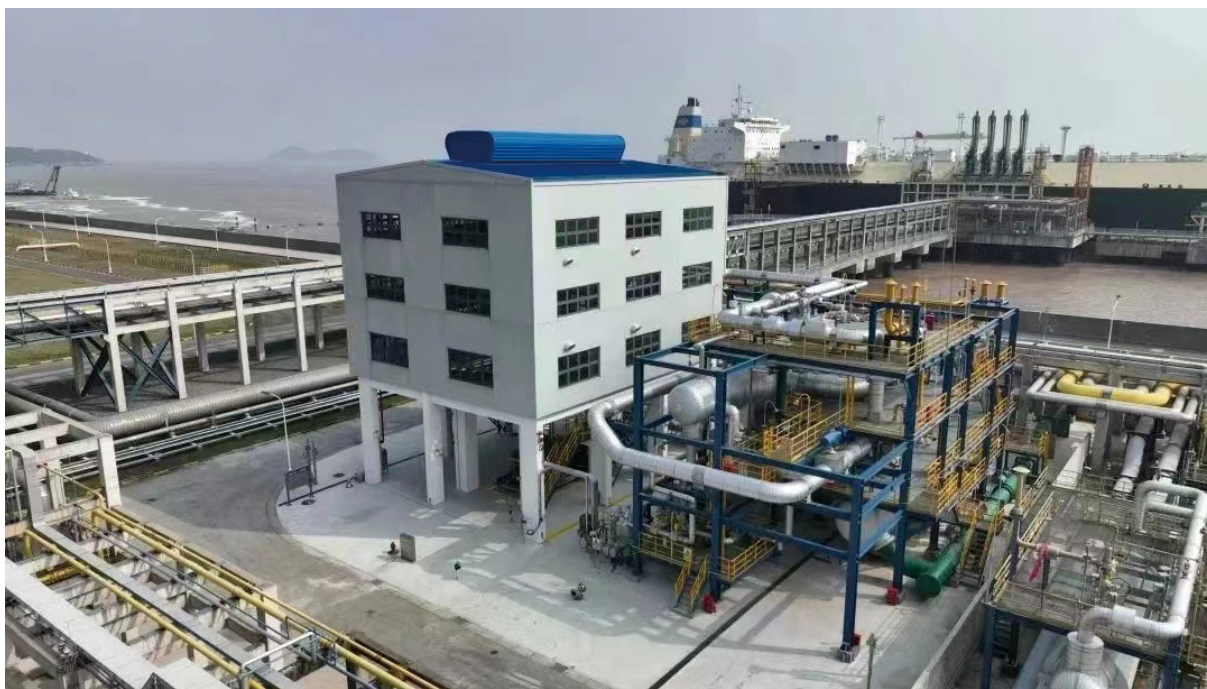
Overall view of Shanghai LNG cold power generation unit
