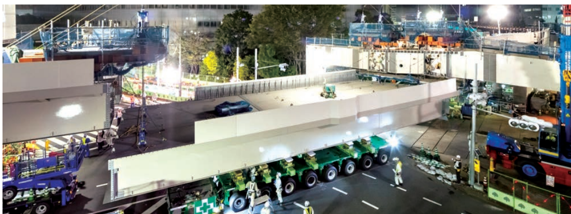
第 31 図 八重洲線汐留高架橋の架替工事 (5) Fig. 31 Shiodome Viaduct reconstruction for the Yaesu Route on the Metropolitan Expressway (5)
