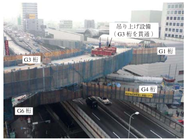
第 17 図 吊り上げ設備 (G3 桁から G4 桁を吊り上げ) Fig. 17 Girder-lifting equipment (G4 girder lifted from G3 girder)
