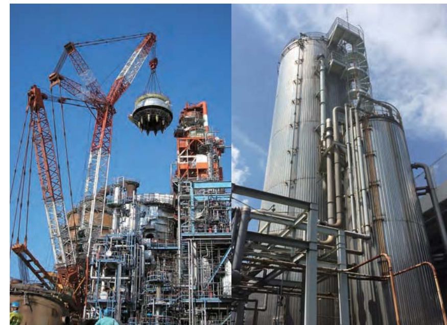
Pressure vessels / Wastewater treatment facility
