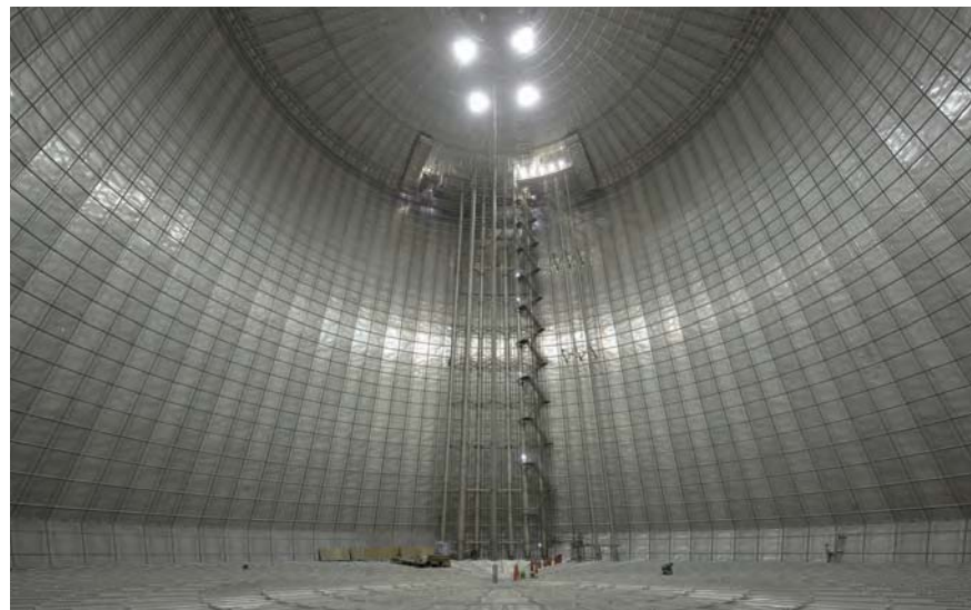
Membrane of world's largest underground LNG tank Photo courtesy of Tokyo Gas Co., Ltd.
