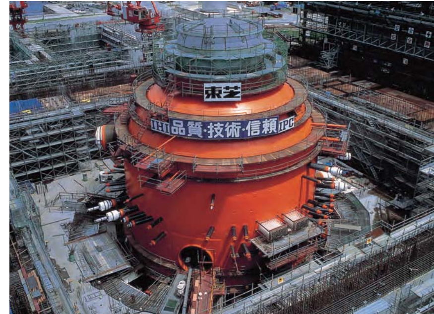
Reactor containment vessel and heavy structures
