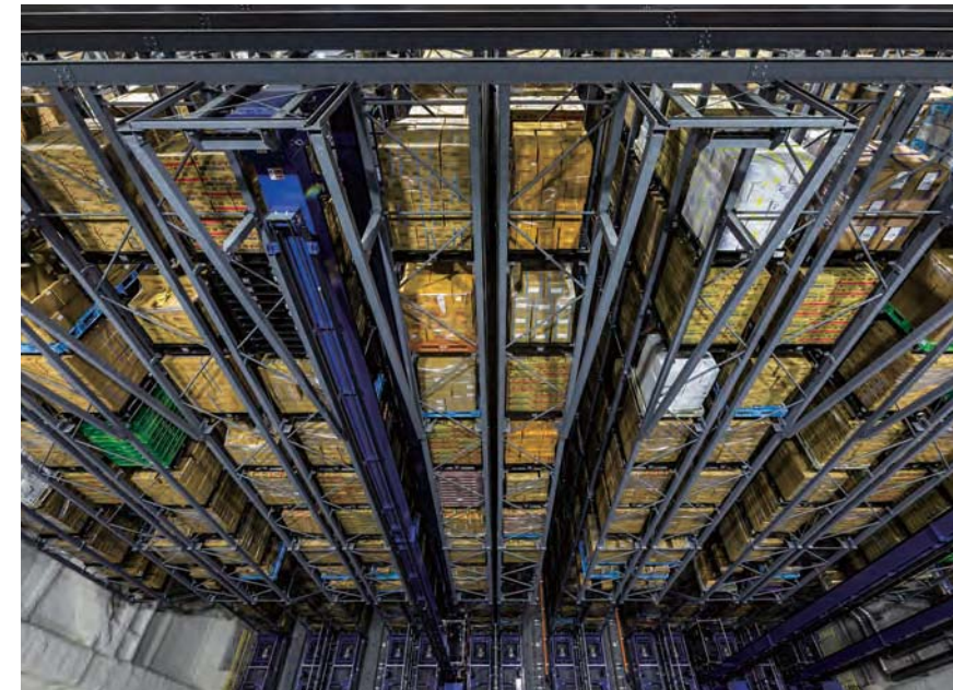
Freezer automated storage and retrieval systems
