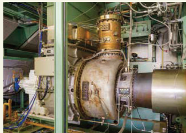
2,000-kilowatt-class gas turbine co-firing liquid ammonia and natural gas at IHI Yokohama Works
