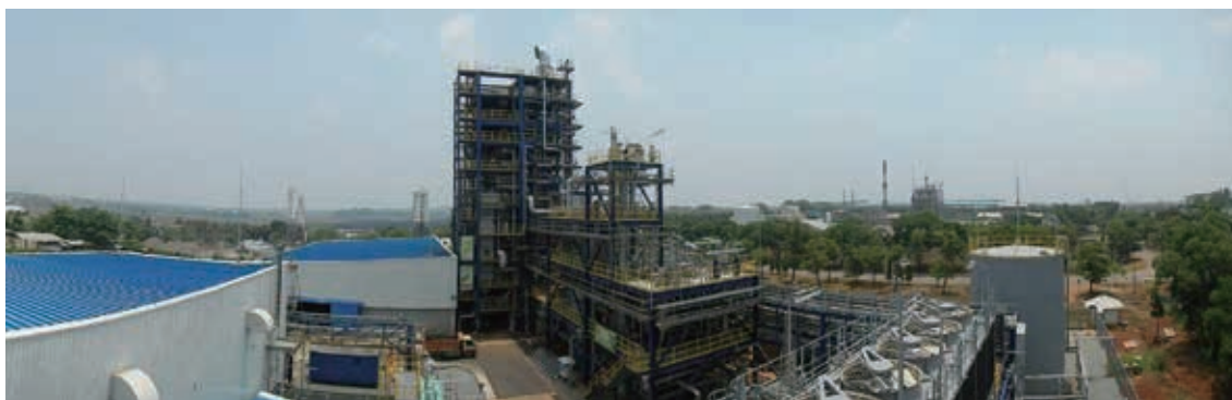
Full view of the demonstration plant (50 t/d) in Indonesia (TIGAR ® gasifier structure seen in the center)
