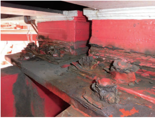
Fig. 4 Corrosion condition at upper chord of floor truss
