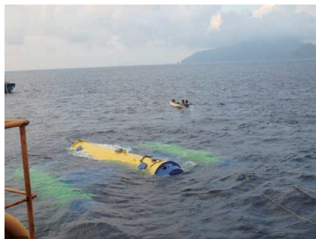
Installation of Kairyu at the site off the coast of Kuchinoshima Island
