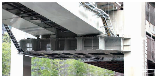
Fig. 3 Lower portion of Pier C4060 : Additional support beam and full-webzation of the box girder
