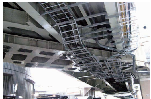
Fig. 4 Pier C4056 : Additional support beam with low height and a bevel angle
