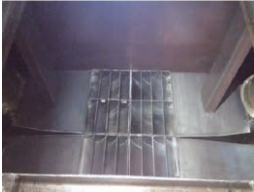
Duct inside the oil tank
