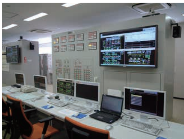
LNG terminal operational training simulator
