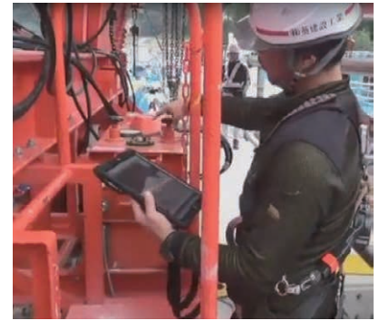
(c) Set up the traveling platform according to the position information shown on the tablet terminal
