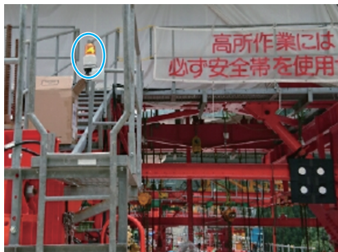
(a) Rotating beacon light for movement monitoring during construction activities
