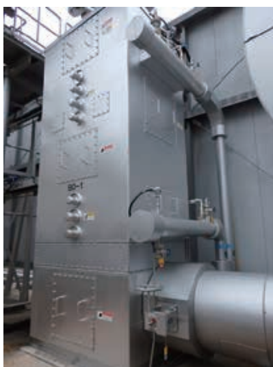
Fig. 2 Exhaust gas boiler
