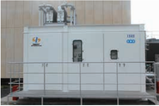
Fig. 4 Enclosure for the ORC and control
