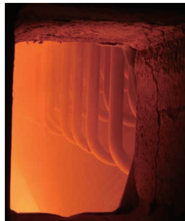
A view inside furnace of 700°C-class superheater
