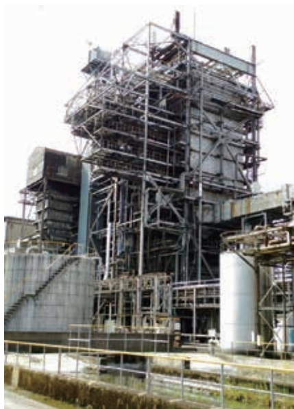
The facility for 700°C-class boiler verification test at the Mikawa Power Plant of Sigma Power Ariake
