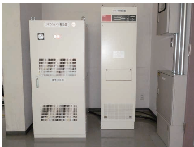
Lithium-ion battery (left) and power management equipment (right)
