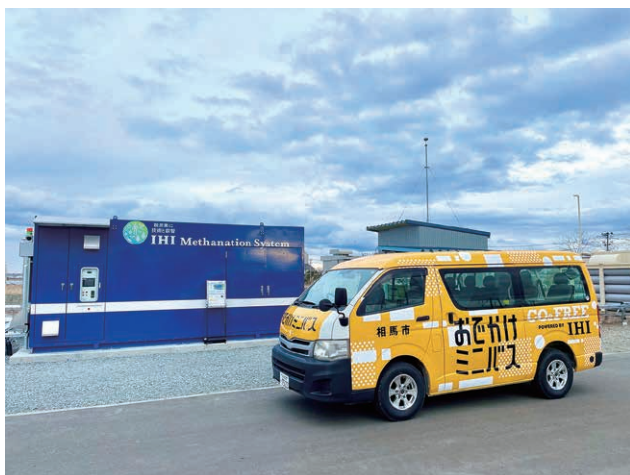
Methanation equipment and the community bus
